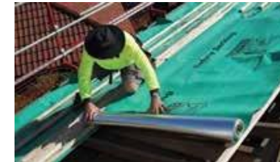
3. SARKING INSTALLED Optional, but recommended. Sarking provides insulation and reflects up to 95% of radiant heat entering the roof.
