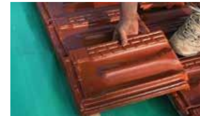
6. TILE INSTALLATION STARTS Tiles are laid sequentially up the roof from the gutter line. Fixing clips or nails are used to secure the roof tiles to the roof.
