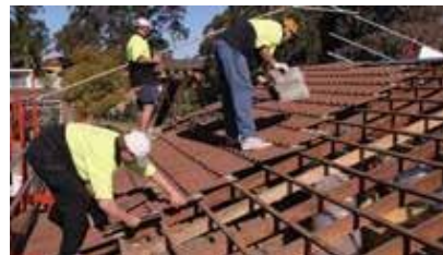
2. OLD TILES & BATTENS REMOVED The old tiles, ridges and battens are removed. Care is taken over existing ceilings and fixtures.
