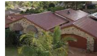
9. COMPLETION Guardrail is removed, the site is cleaned, and any leftover roof tiles are removed.
