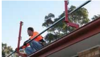
1. SAFETY RAIL INSTALLED IF REQUIRED Safety is paramount. Guardrail is installed around the roof to protect roof tilers and your family.
