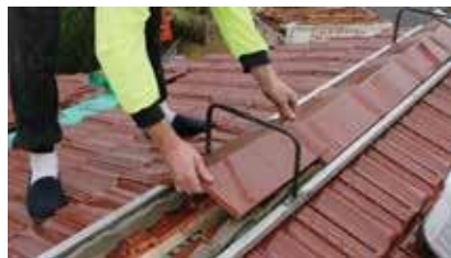
7. RIDGE TILES INSTALLED Ridge tiles are secured and bedded in place using Roof Pointing mortar.
