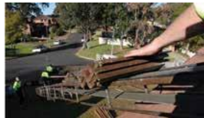
5. NEW TILES TRANSPORTED TO ROOF Conveyors transport new roof tiles to the roof.
